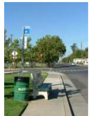
View west toward Rio Linda Elementary School showing narrow sidewalks and lack of space for transit stop amenities.
